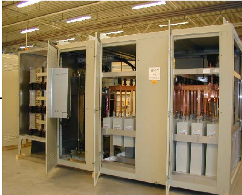
Direct Electric Heating Toppersides
